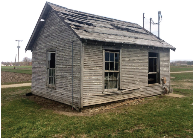
Figure 7. Shed previous condition. Taylor M.
